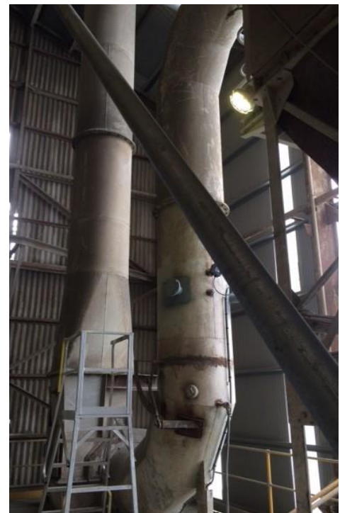
Figure 2: Cement Mill 2 Exhaust Duct
